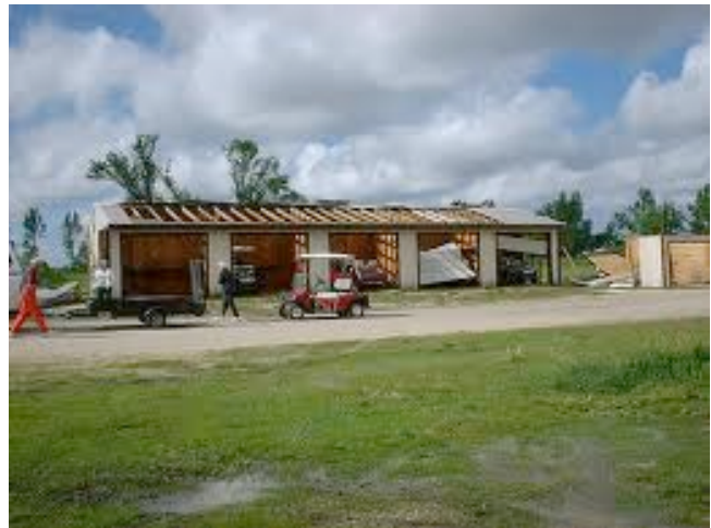
Picture above: The effect of wind damage to a golf cart storage shed.
